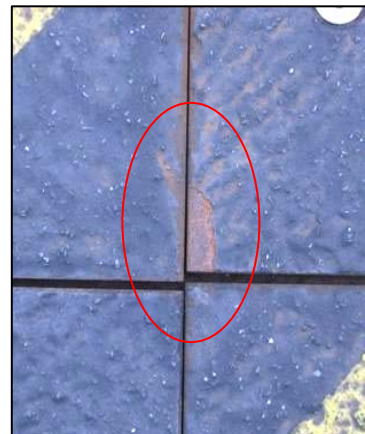
Figure 3: Surface treatment chipped at corners.
